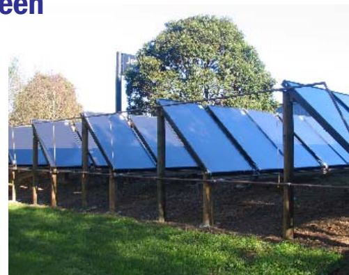
The solar panel farm at Jet Park
